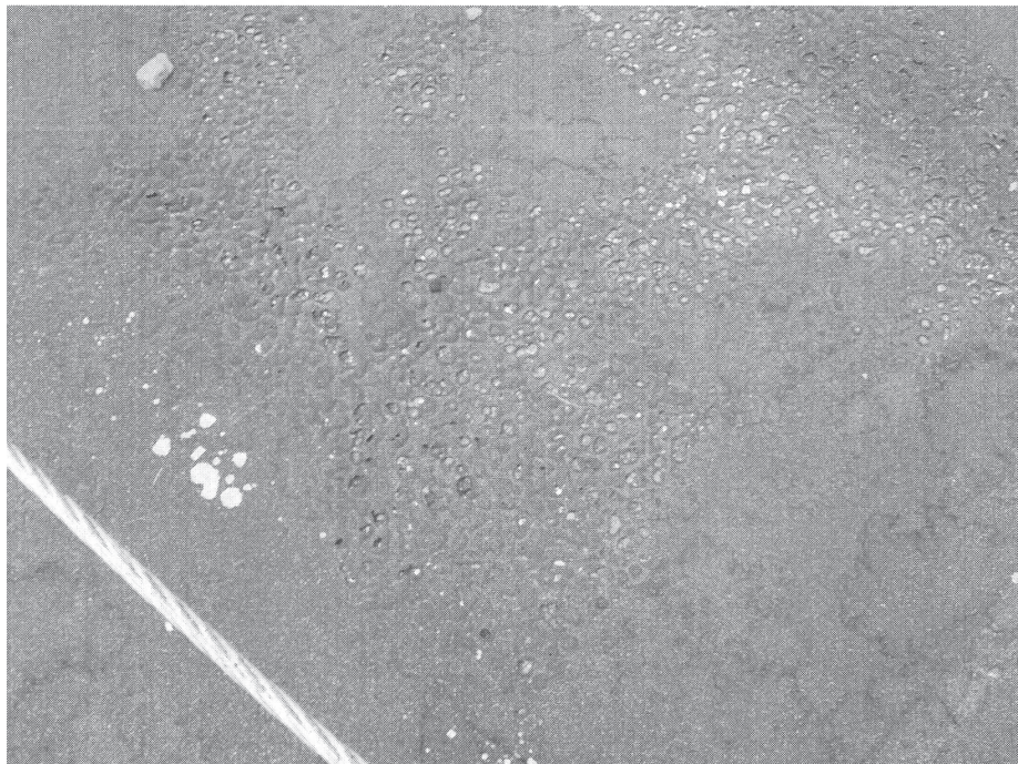
Figure 2: Sags (craters) in top surface bitumen material layer
