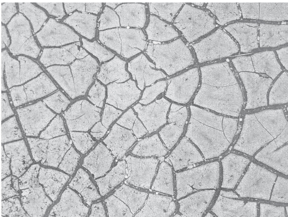
Figure 4: Disordered network of deep cracks in top surface bitumen material layer.
